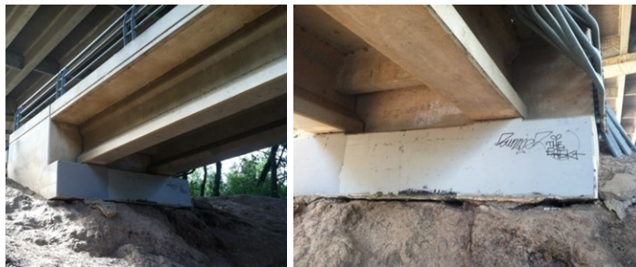
Figure 20. Hangout 2 Under the Structure of Small Bridge that Pass Across the Lake. This hangout was detected under the structure of the small bridge that is used to pass across the lake.
